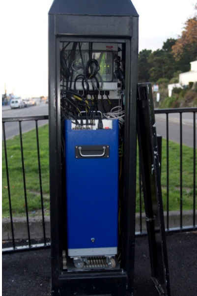
Figure 4: A POD device installed at Marine Parade.
