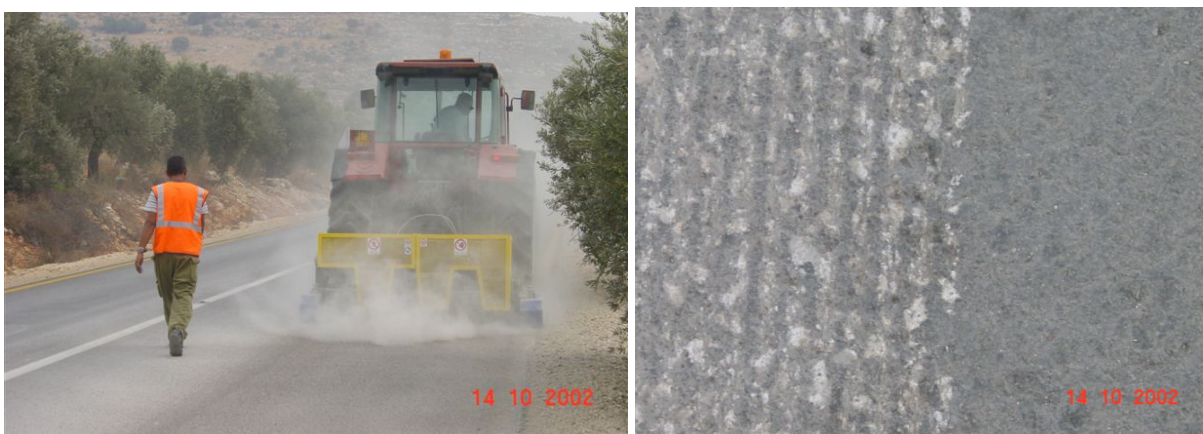
Figure 16: The Rotating Discs process at work and the attained surface
