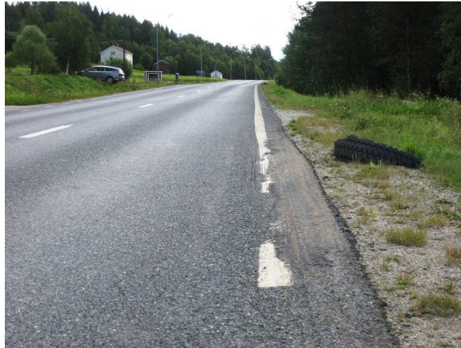
Figure 9 Edge deformation at HS Åkerö. Take note of the exploded truck tyre!
