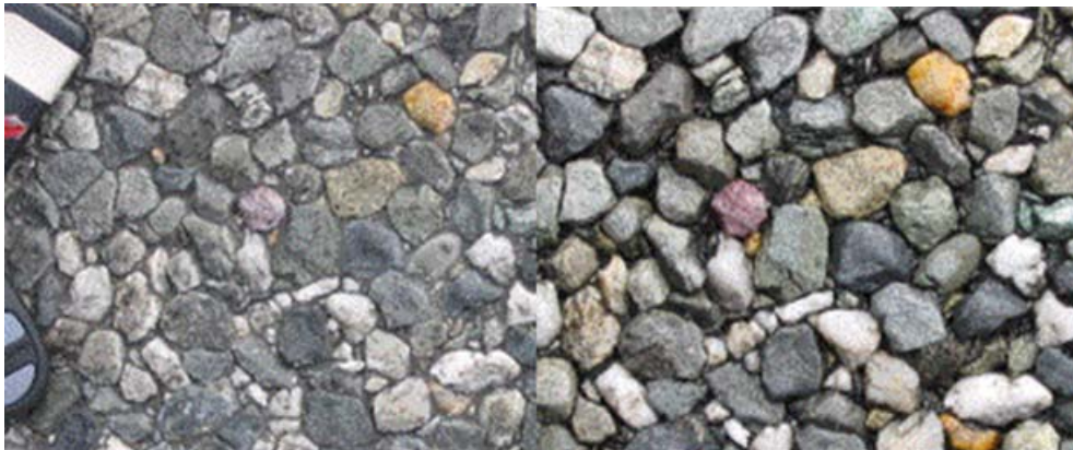
Figure 6: Polished Aggregate before (on left) and after (on right) Ultra High Pressure Watercutting.
