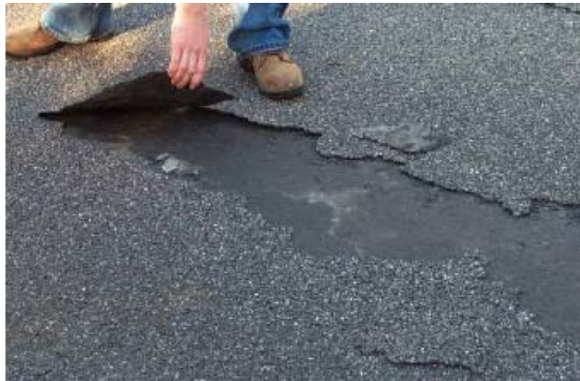
Figure 3: Delamination on Wainuiomata Hill.
