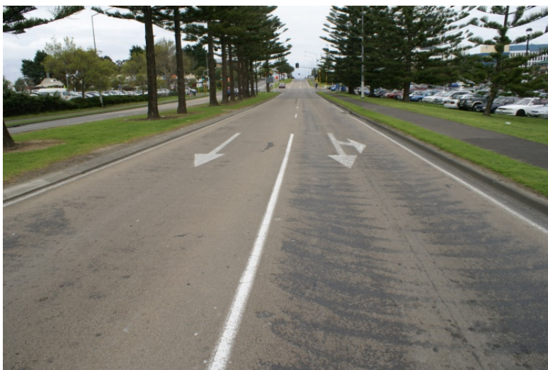
Figure 2: Poor binder application causing chip loss.
