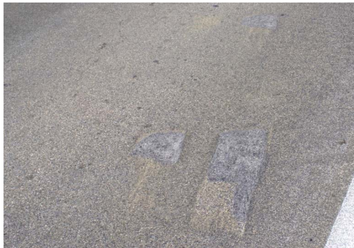
Figure 1: Traffic too early.
